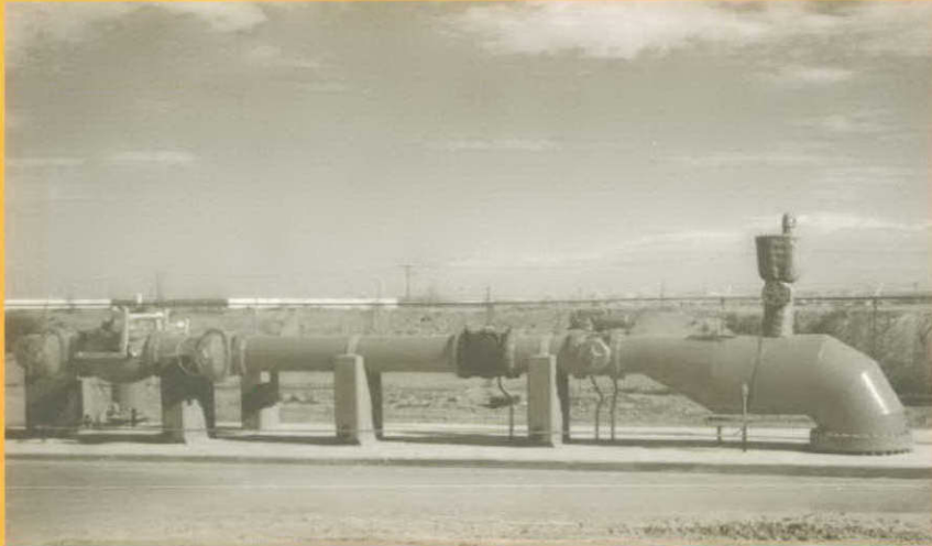
Booster station for the Lower Valley Project
