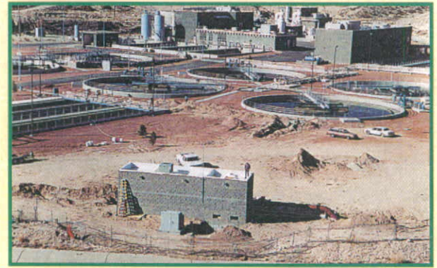
View of Northwest Wastewater Treatment Plant and pumping station for the reuse project of reclaimed water
